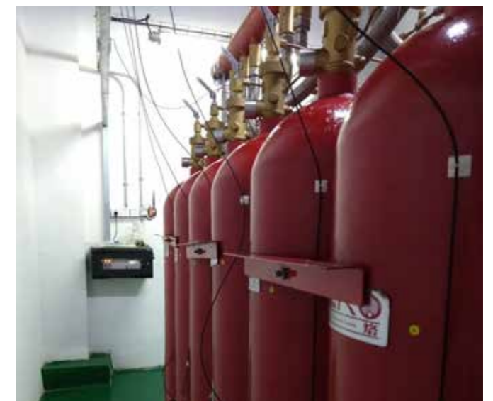
▶ Permalevel® MULTIPLEX installed in a FM200 Cylinder Room.
