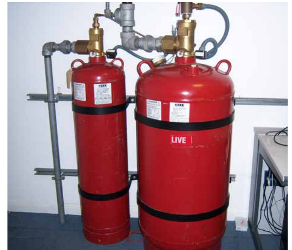
▲ FM200 Cylinders at a Power Plant.
